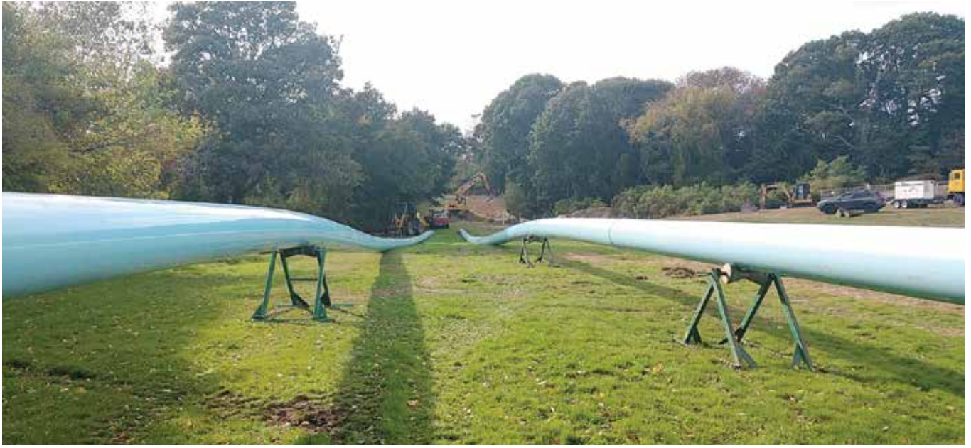
Fusing of PVC pipe segments was done at the golf course on the East Providence side of the river
