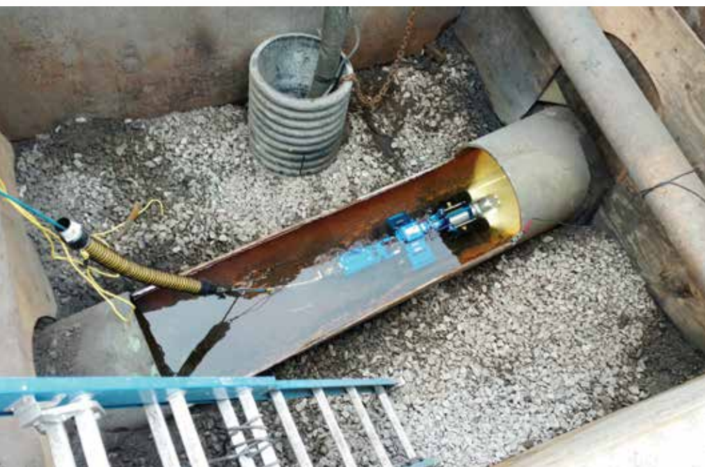
CCTV inspection of the main was critical to identifying the location and nature of the leak
