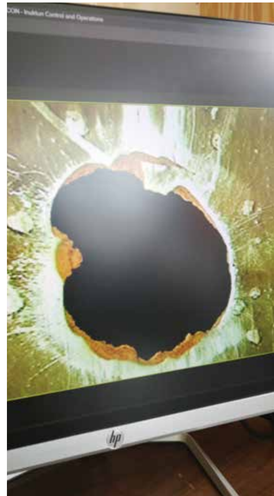
Two holes were found in the 24-inch steel pipe in bedrock approximately 170 feet beneath the surface of the Providence River
