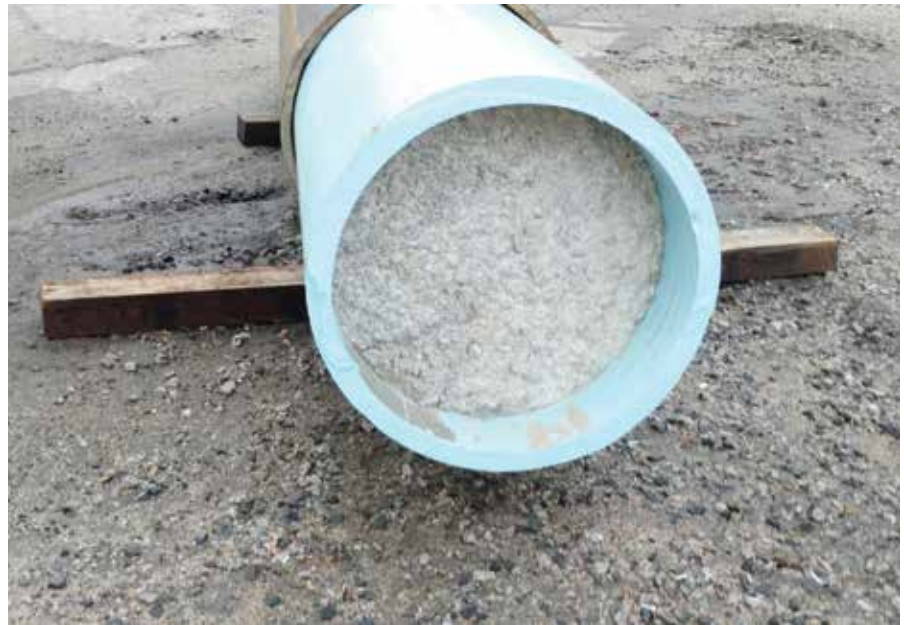
Pull head needed to be watertight so a concrete plug was fused onto the first section of pulled PVC pipe
